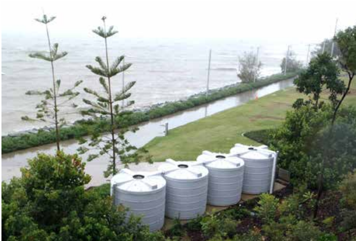
Send the treated stormwater to tanks for irrigating a neighbouring park. Location - Marine Parade, Redcliffe
