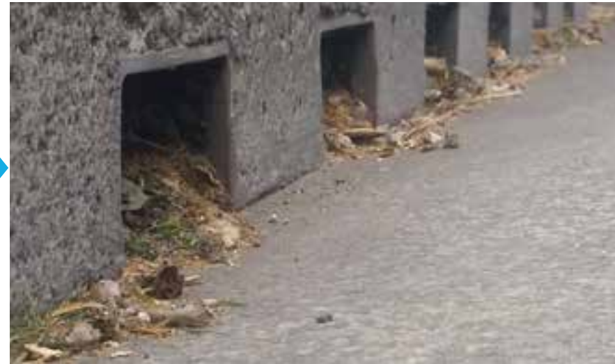
Problem: Inlets become blocked with sediment and leaf litter
